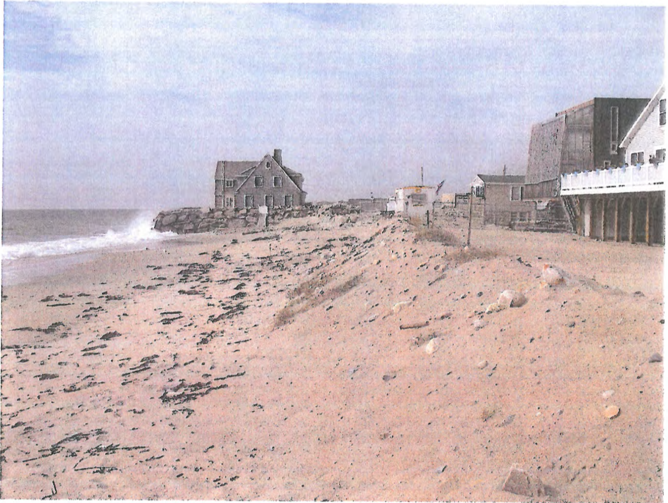
Figure 3. The recently restored dune/dike on the property located east of the proposed experimental coastal erosion control technique. The proposed structure will tie into the rock structure and align with the dune/dike to the east.
