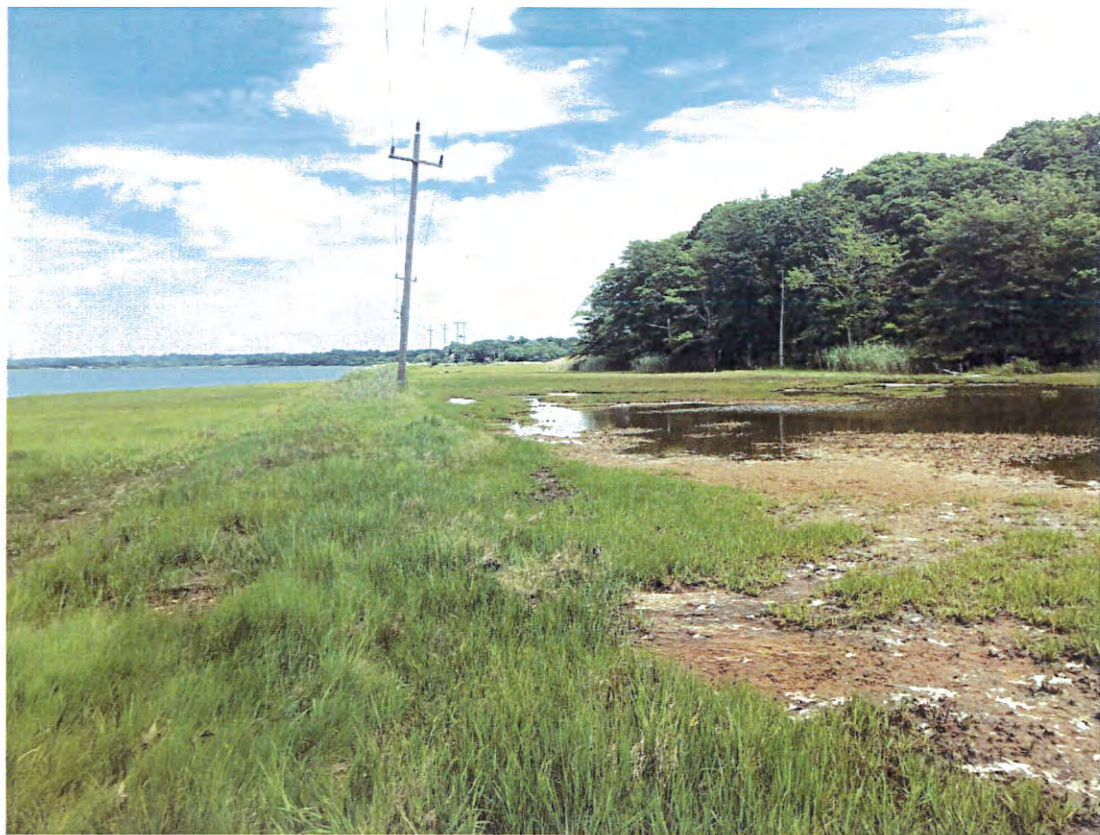
Figure 7: Berm impounds standing water on the marsh platform causing vegetation die-off.
