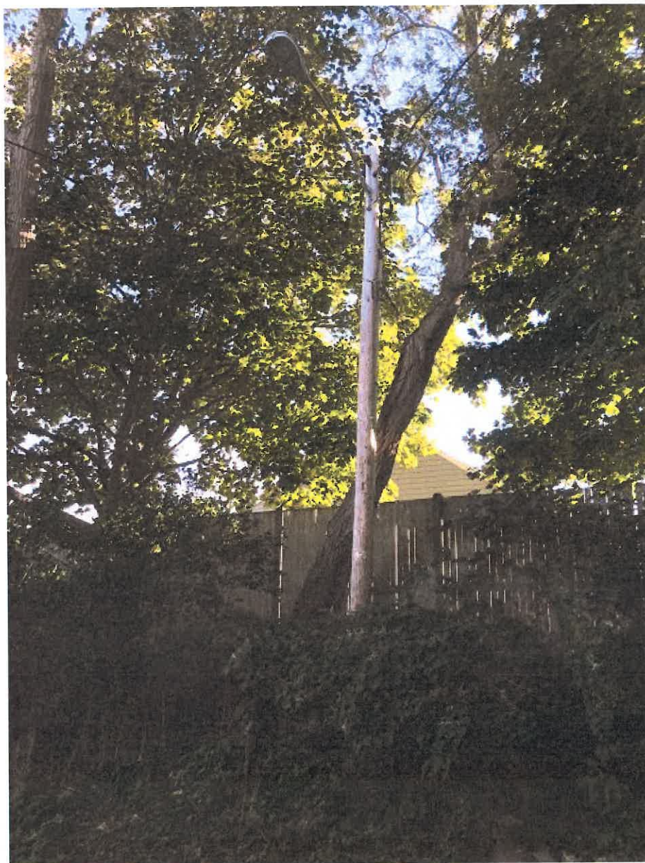
Figure 6: One of the power poles along East Power Street
