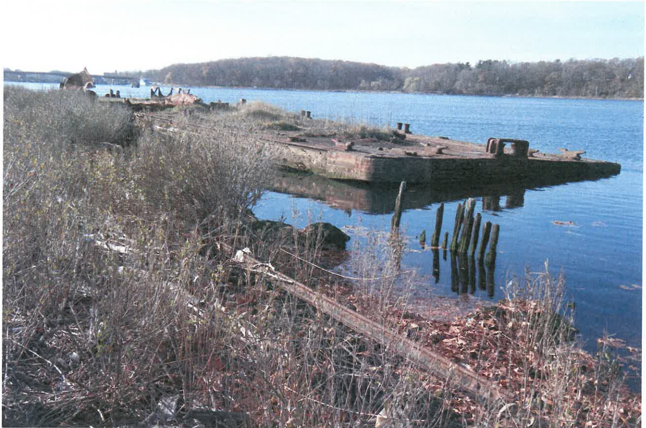
Photo 17: Deteriorating barge to be removed
