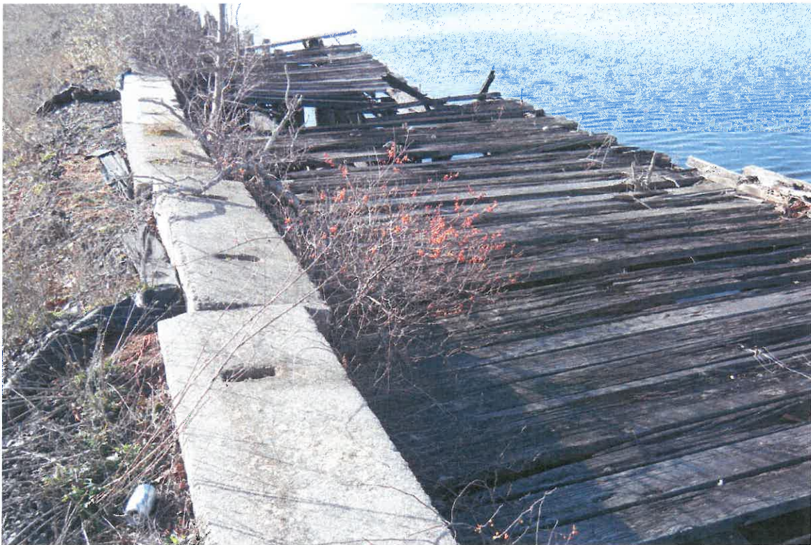
Photo 14: Deteriorating coastal decking
