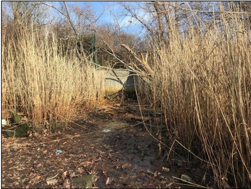
Photo 3: Concrete headwall and 18" outfall at North Landfill, between A 72 and A73 (looking east)
