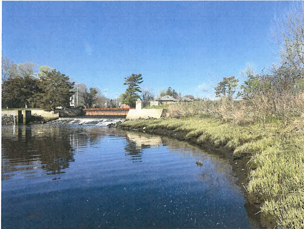
Photo 1: View of the Lower Kickemuit Dam and adjacent salt marsh facing west toward the dam.
