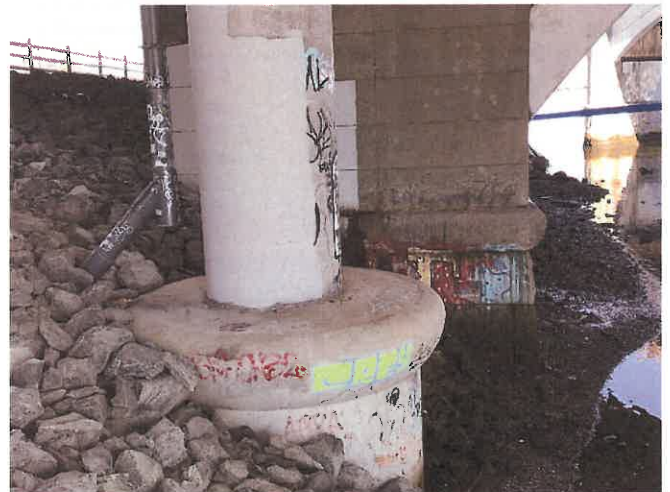
Photo 15. Northerly view of shoreline, where rip rap meets tidal waters between the EB and WB foundations, representing sole location under bridge where concrete walls are not present. Column in foreground is that shown as last column in Photo 14, abutting massive pier wall to the north.
