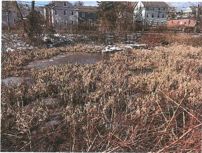
Photo 26. Northwesterly view of Sedimentation Basin, the upper of the three Gano Street water quality ponds, indicating extent of sediment accumulation.
