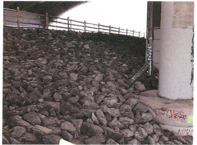
Photo 17. Northwesterly view of slope protection, as taken from concrete bridge structures and looking upslope towards split-rail fence along Bikeway.
