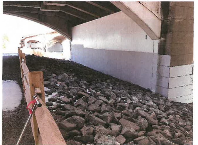
Photo 19. Northerly view of rip rap slope protection shown as opposing view as that in Photo 18. The full extent of the WB pier wall and presence of landward rip rap is shown. For reference, the pier is the same as that shown in Photos 14 and 15.
