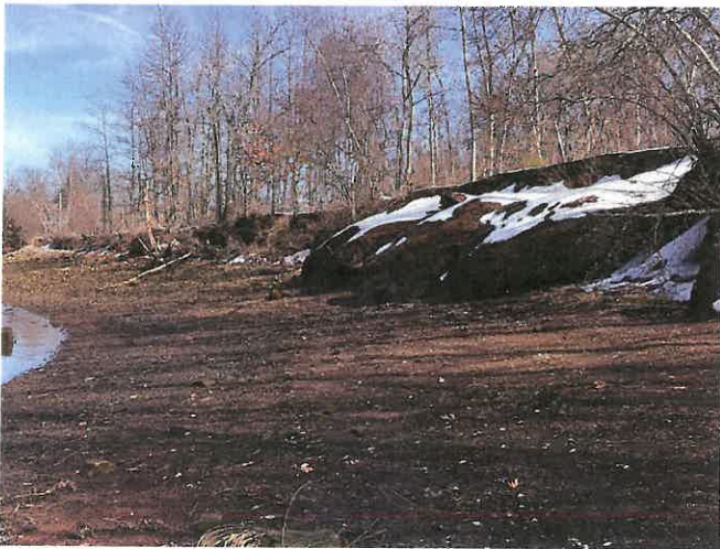
Photo 9. North/northeasterly view of elevated, artificial landforms along the northerly portion of the delineation. The feature edge was delineated at the top of the landforms, along the eroded embankment crest.
