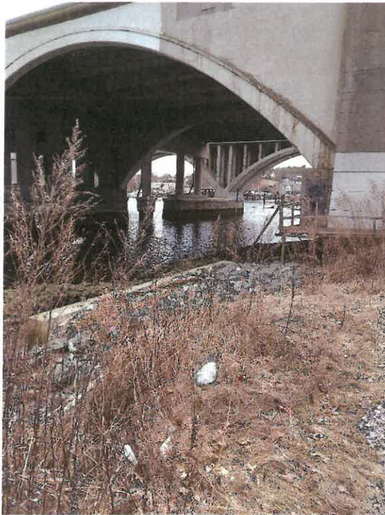
Photo 3: Coastal Feature #4 (Concrete structure / deteriorating rip rap) at northwest corner of bridge. See Figure 2.
