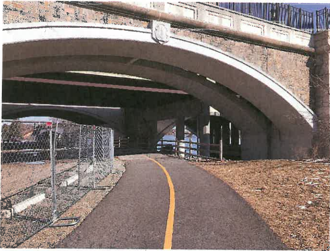
Photo 35. Northerly view of Bikeway approach to Washington Bridge. The Gano Street and Bikeway Relocation will occur under this span. Note the elevated topography at right to separate the project from the Hunter S. Marston Boathouse, located out of the viewport to the immediate right.
