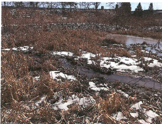
Photo 28. Southeasterly view of severe sediment accumulation, as taken from western inlet. The Gano Street Off-Ramp is visible in background.
