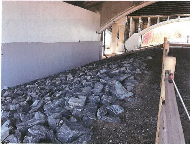
Photo 18. Southerly view of slope protection present landward of the massive WB pier wall.
