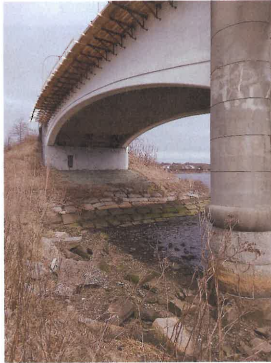
Photo 1: Coastal Feature #1 (Concrete block revetment) and Coastal Feature #2 (Deteriorating rip rap) at northwest corner of bridge. See Figure 2.
