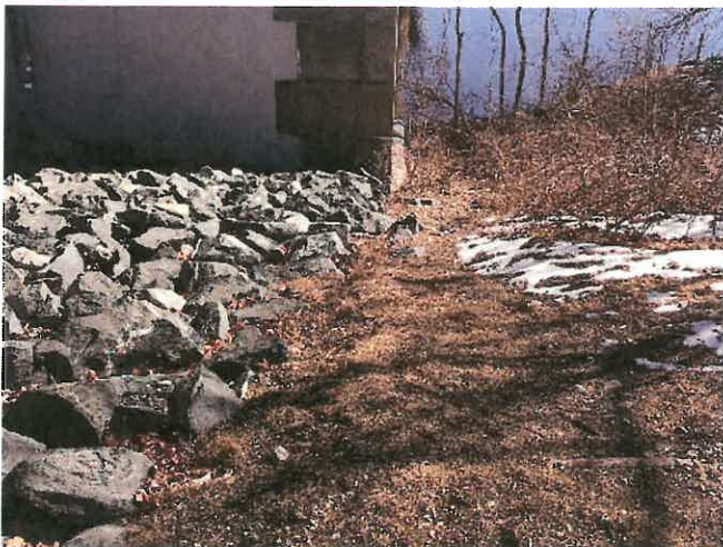
Photo 20. Easterly view showing southerly extent of rip-rap slope protection as being limited to footprint (dripline) of the bridge deck above. As indicated in the document, the rip-rap slope protection appears as a rectangular area extending landward of the Manmade Shoreline.
