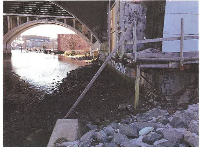
Photo 11. Similar view as in Photo 10 but taken from a vantage point further north to show the complete length of the foundations.
