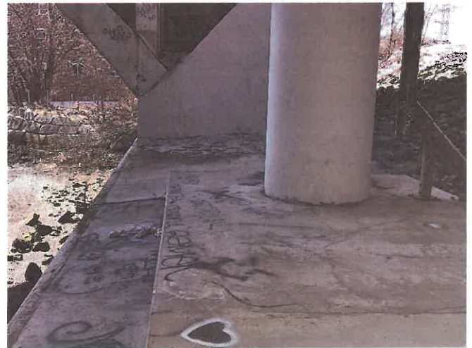
Photo 13. Southerly view of abutment shown in Photo 12 but shifted slightly landward to show massiveness of foundations and adjoining rip rap slope protection to the right.
