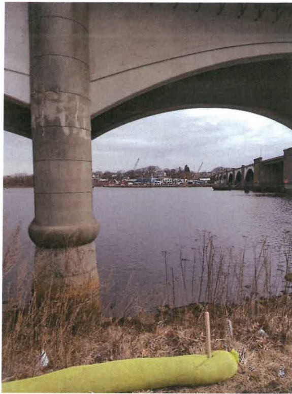
Photo 7: Looking across the channel to Coastal Feature #9 (Rip rap) at the northeast corner of the bridge. See Figure 3.
