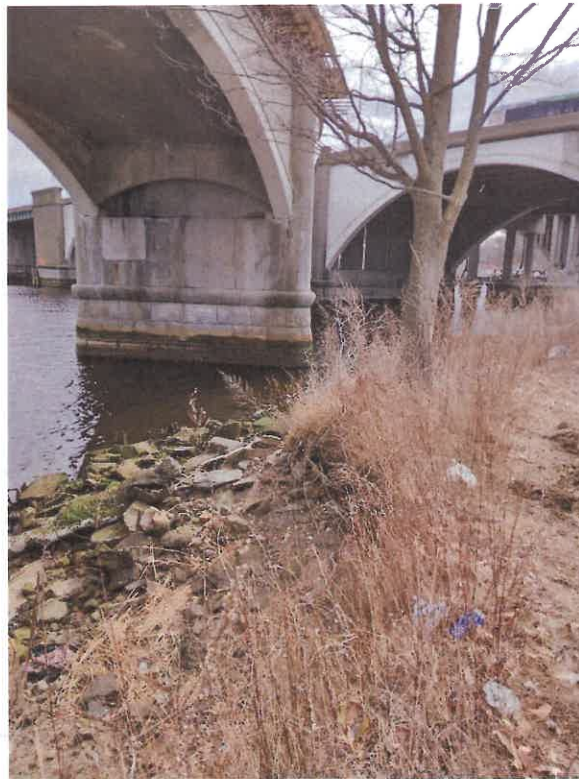
Photo 2: Coastal Feature #3 (Eroding bank) at northwest corner of bridge. See Figure 2.
