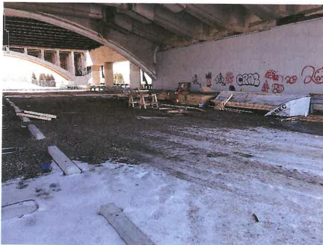
Photo 39. Southwesterly view under Washington Bridge to show the barren substrates on which the Gano Street Relocation will occur. The I-195 WB span is in the foreground.
