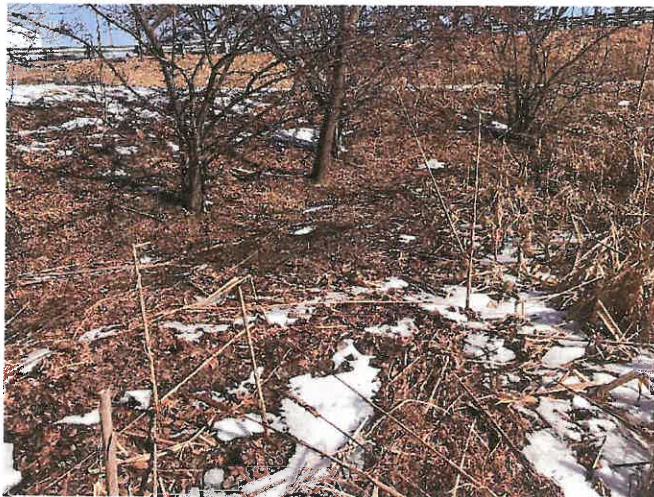
Photo 30. Northeasterly view along northern edge of Sedimentation Basin showing how the depth of sediment accumulation has overtaken the original basin side slope and is nearly even in elevation with original woody landscape plantings.
