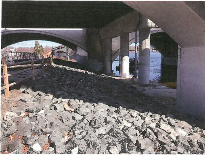
Photo 16. Northerly view of rip-rap slope protection abutting massive concrete bridge structures and extending upslope to Blackstone River Bikeway.
