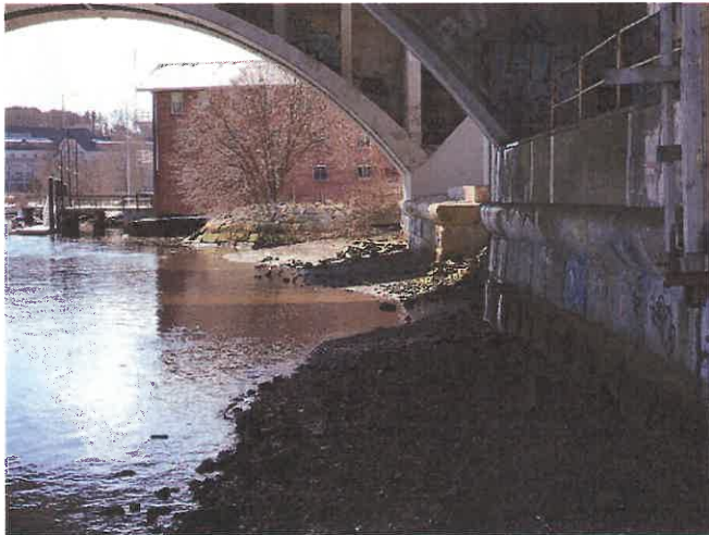
Photo 10. Southerly view under the Washington Bridge, showing I-195 Eastbound (EB) and Westbound (WB) pier foundations, with the Hunter S. Marston Boathouse shown in the background.
