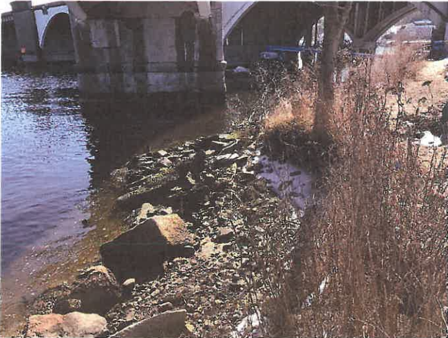
Photo 24. Southerly view of eroded feature edge north of the Bridge. The pier visible near the foreground supports the Gano Street Off-Ramp.
