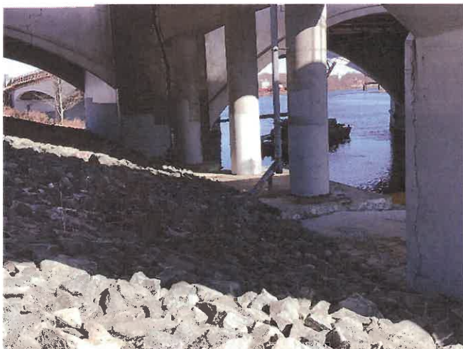
Photo 14. North/northeasterly view of massive foundations, piers, and pier walls forming the Manmade Shoreline. The relationship of the rip-rap slope protection under the Bridge, as referenced in the document, is clearly visible.
