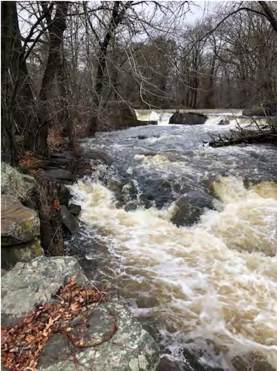
The head cut in the ledge (at high water) located 50' below the entrance to the ladder.
