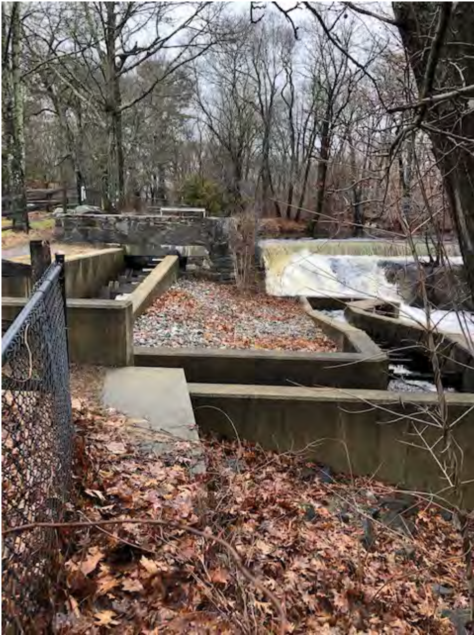
The Hunts Mill Fish Ladder located at the Hunts Mill Dam
