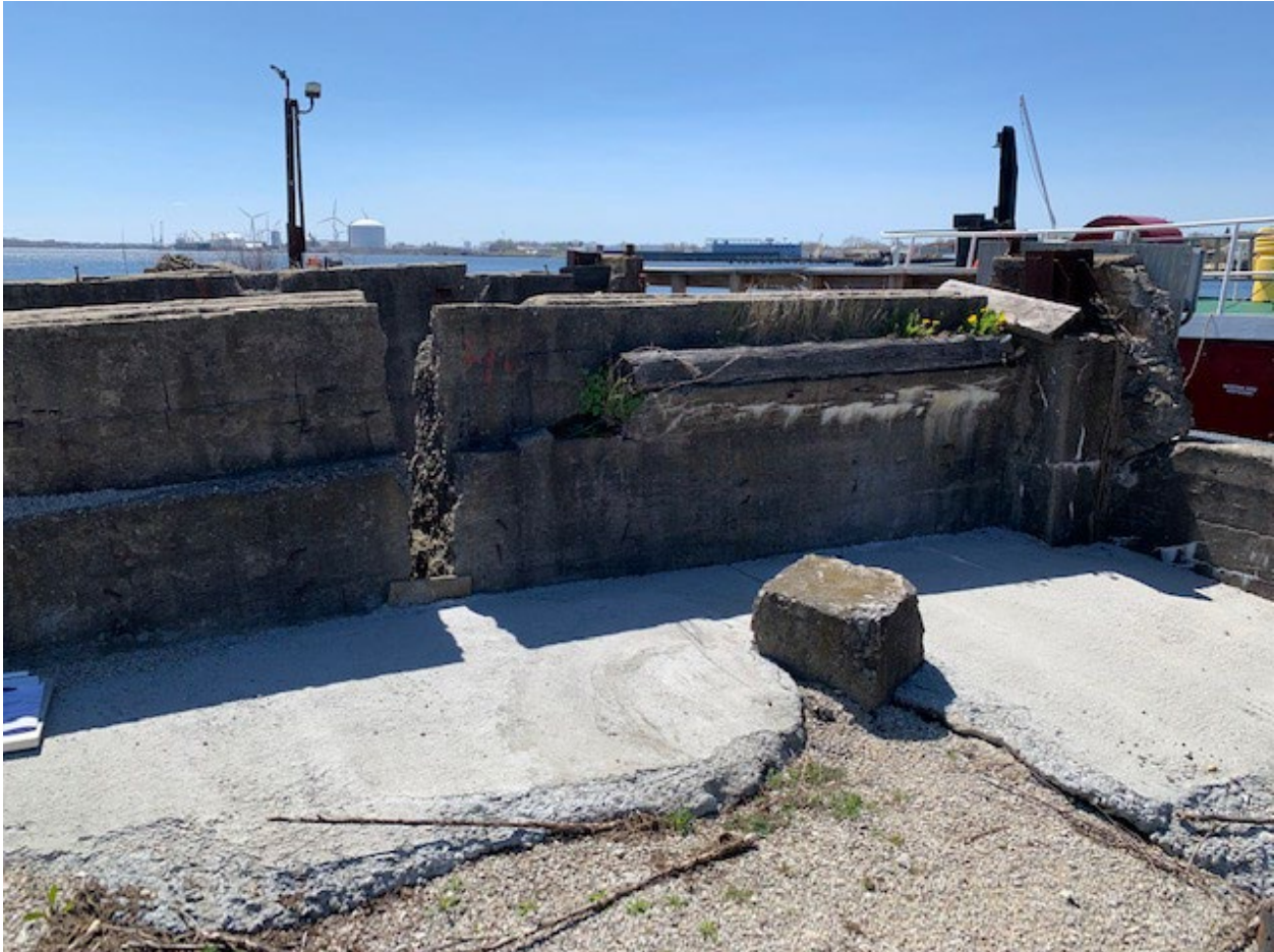
Photo 6: Failure/crack in the north wall of the south concrete pen; displacement indicates differential settlement. Note concrete placed in an attempt to address soil loss into the pen.
