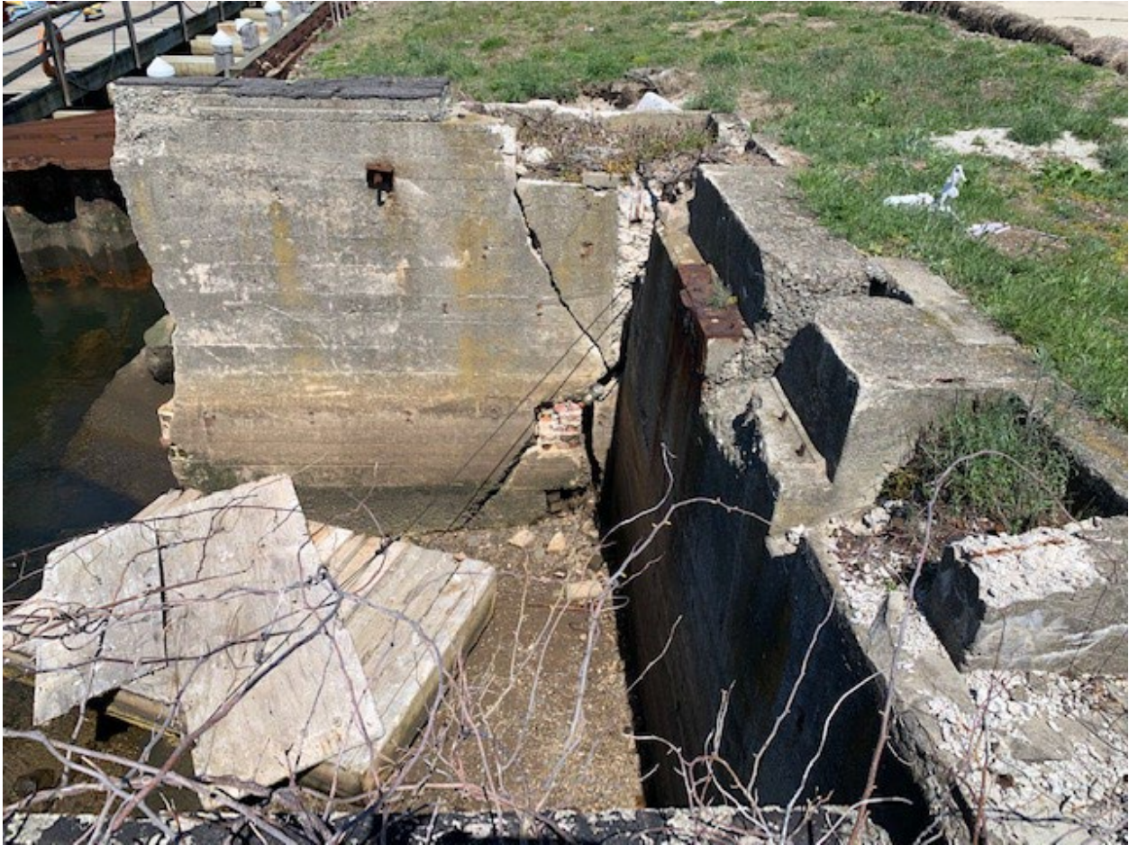
Photo 3: Overview of the north concrete pen; note partial failure and large crack in remaining wall (a portion of this structure (wall & slab) previously failed into the ship berth and required removal). The intent would be to demolish the north wall of this structure, return the proposed sheeting to a point about at the west end of the pen, and extend the existing stone revetment across the pen. This would stabilize the area and remove any future hazards to persons or navigation.
