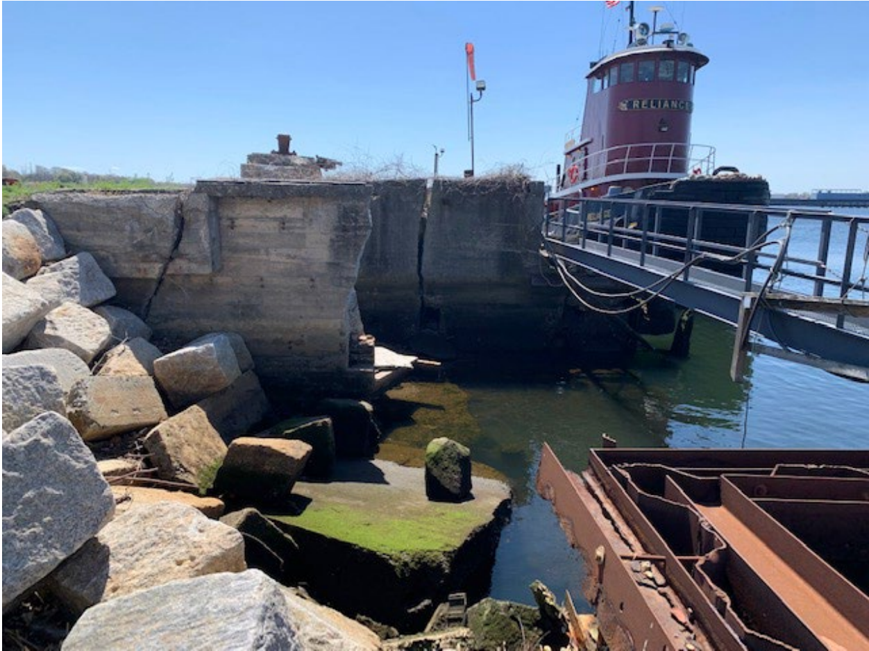
Photo 1: Overview of the north concrete pen; note partial failure and large crack in remaining wall (a portion of this structure (wall & slab) previously failed into the ship berth and required removal). The project would demolish the failed north wall of this structure, construct a stone revetment/rip across the pen floor area to the south wall (generally matching the profile of the existing revetment), and installing sheeting from the bulkhead at the south side of the pen across the opening to the steel sheets at the timber pier (generally aligned to match the aluminum bridge across the area. This work would stabilize the area and remove any future hazards to persons or navigation.
