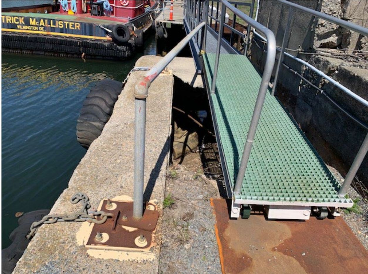
Photo 9: Severe settlement and soil loss adjacent to failing north concrete pen. This condition creates a dangerous condition at the support/landing at the pedestrian bridge used to access the south tug berth.
