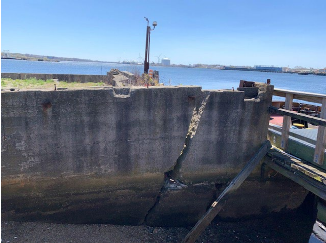
Photo 5: Failure/crack in the south wall of the south concrete pen; displacement indicates differential settlement across the pen. The intent would be to demolish the top few feet of this structure, extend the stormwater outfall through the steel sheetpile bulkhead , and backfill the area level with the adjacent ground. This would stabilize the area and remove any future hazards to persons or navigation.
