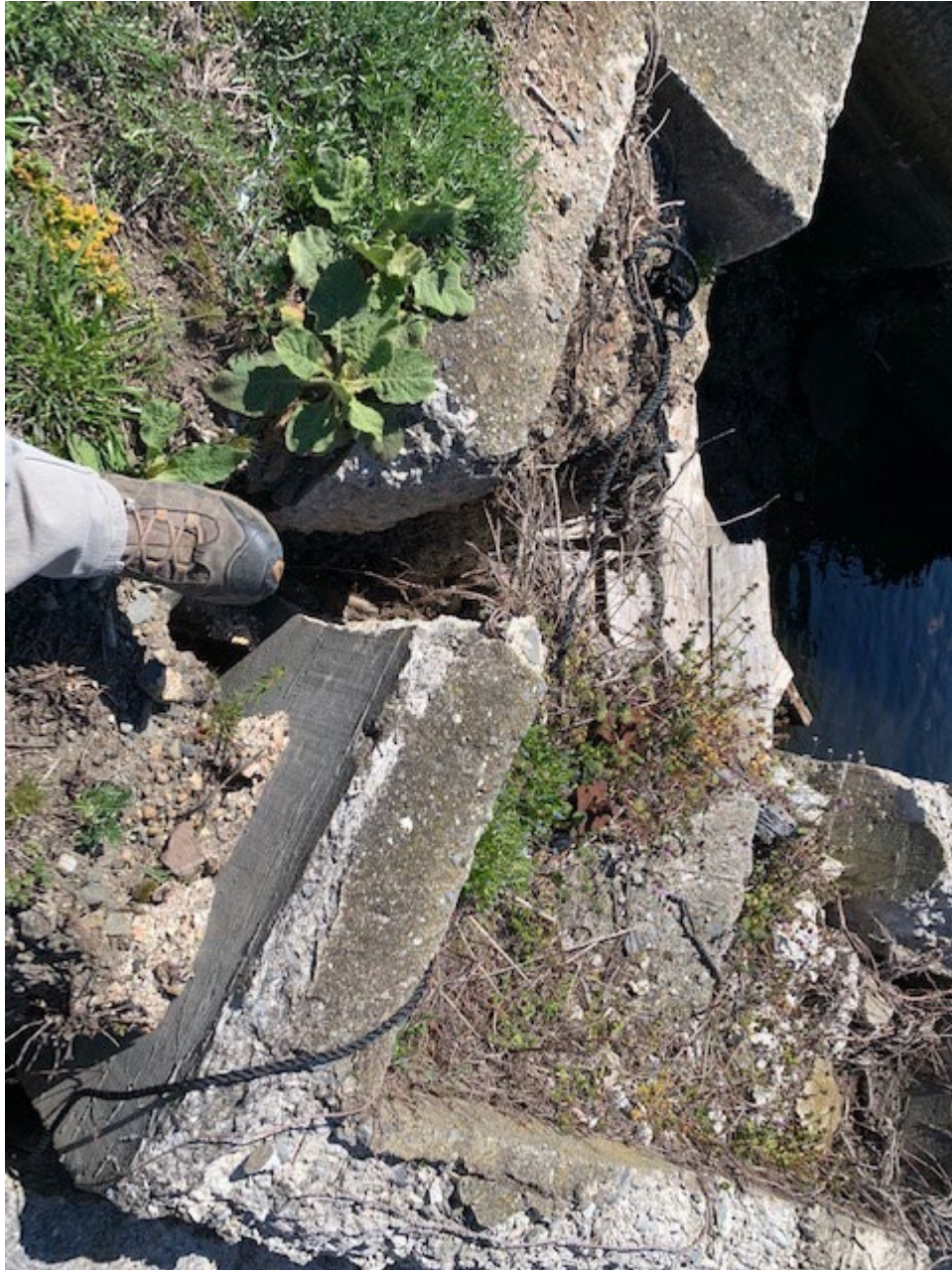
Photo 2: Large crack and displacement in back wall of north pen
