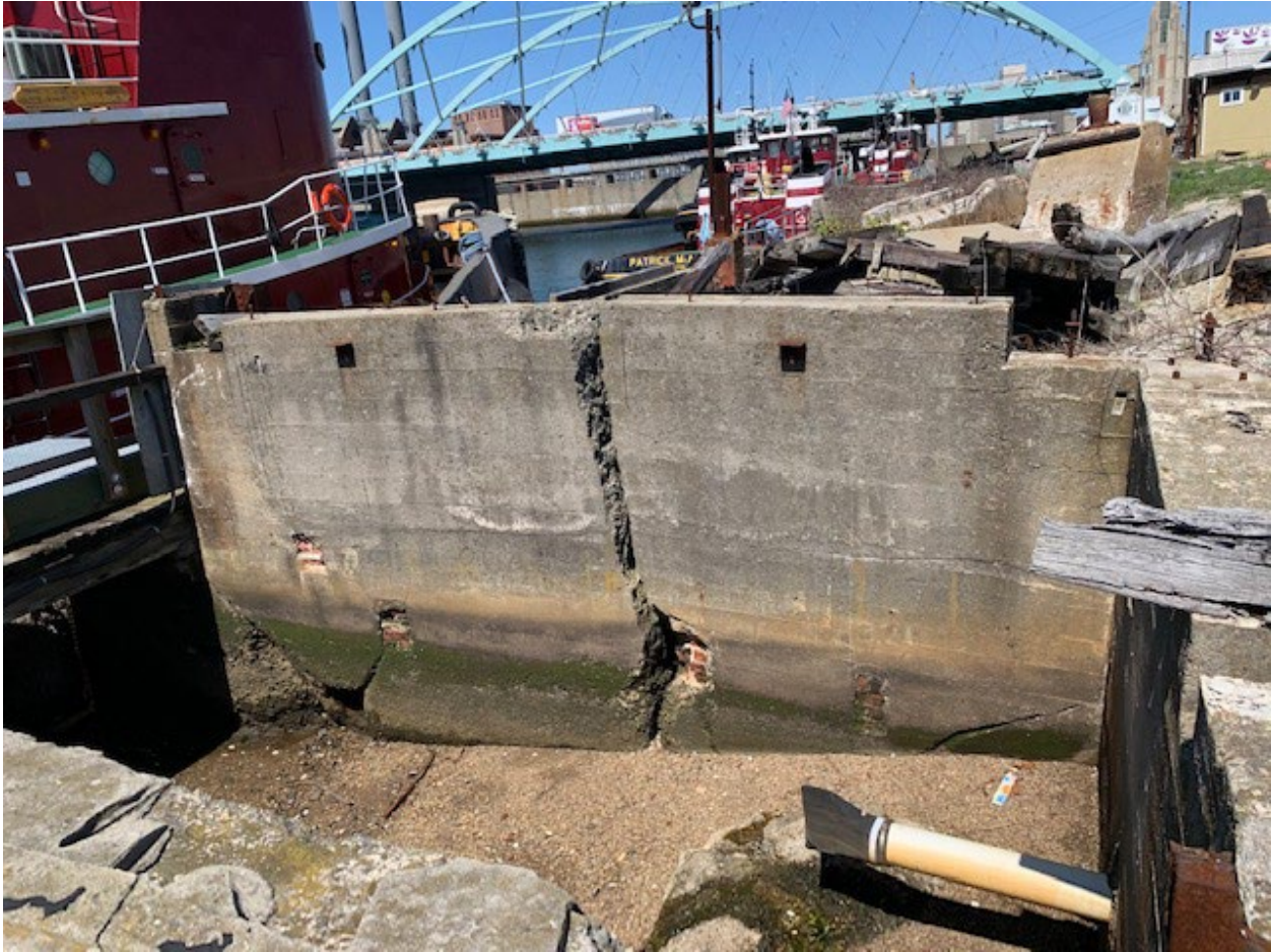
Photo 7: Failed north wall of the south concrete pen and 8" dia. stormwater outfall with duckbill valve. The intent would be to extend this outfall pipe through the steel sheetpile bulkhead. The mean high tide line was determined at this site from the black staining on the concrete walls. The soil above the concrete floor at the western end of the pen is believed to be the result of erosion of the upland soil through the large cracks in the pen walls.
