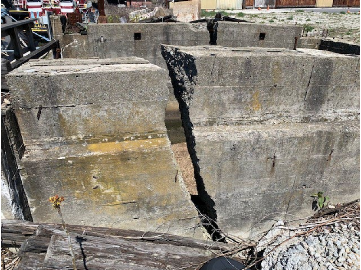
Photo 8: Close view of failure in south wall of the south concrete pen
