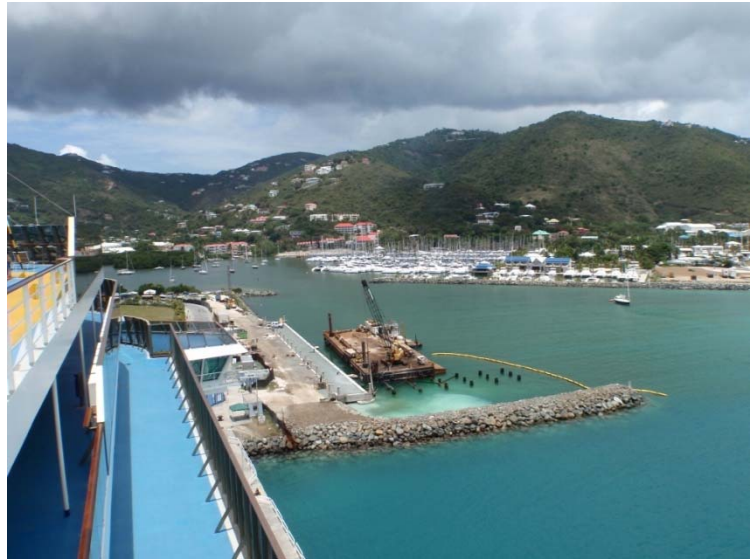
Tender Landing, Breakwater and Piles for Ferry Dock During Construction – Breakwater in
