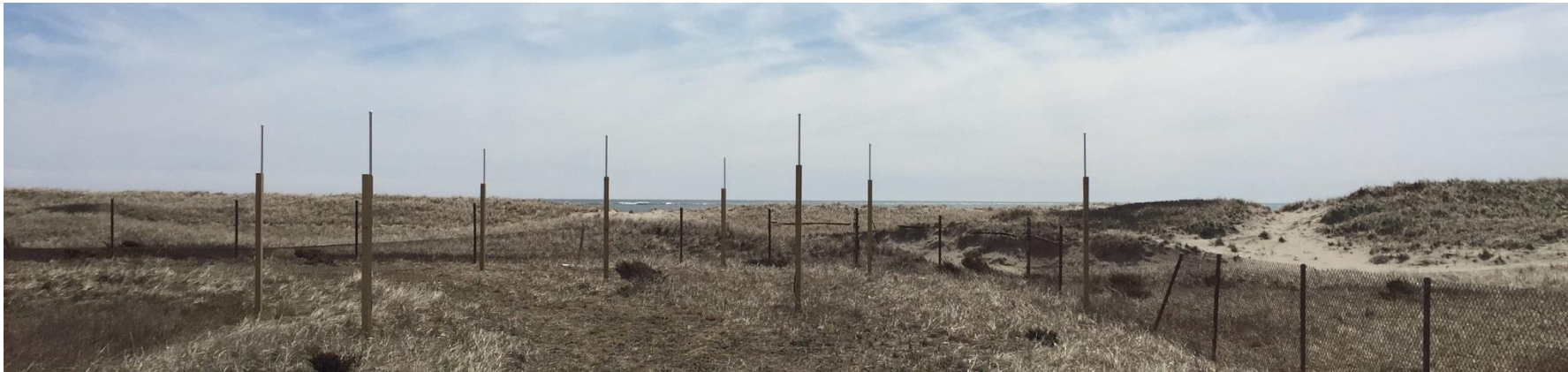
UH HFR receive antenna installed on Nantucket Island, MA.
