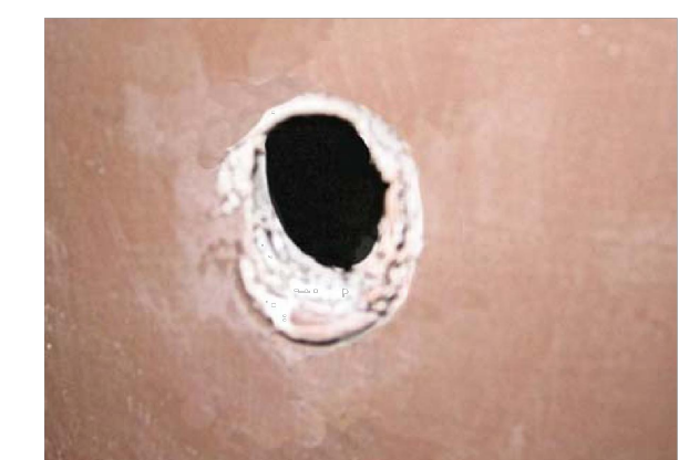
Bolt Hole Elongation - exterior
