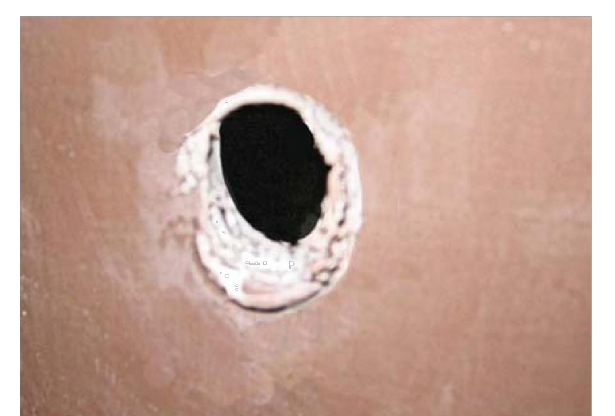
Bolt Hole Elongation - exterior
