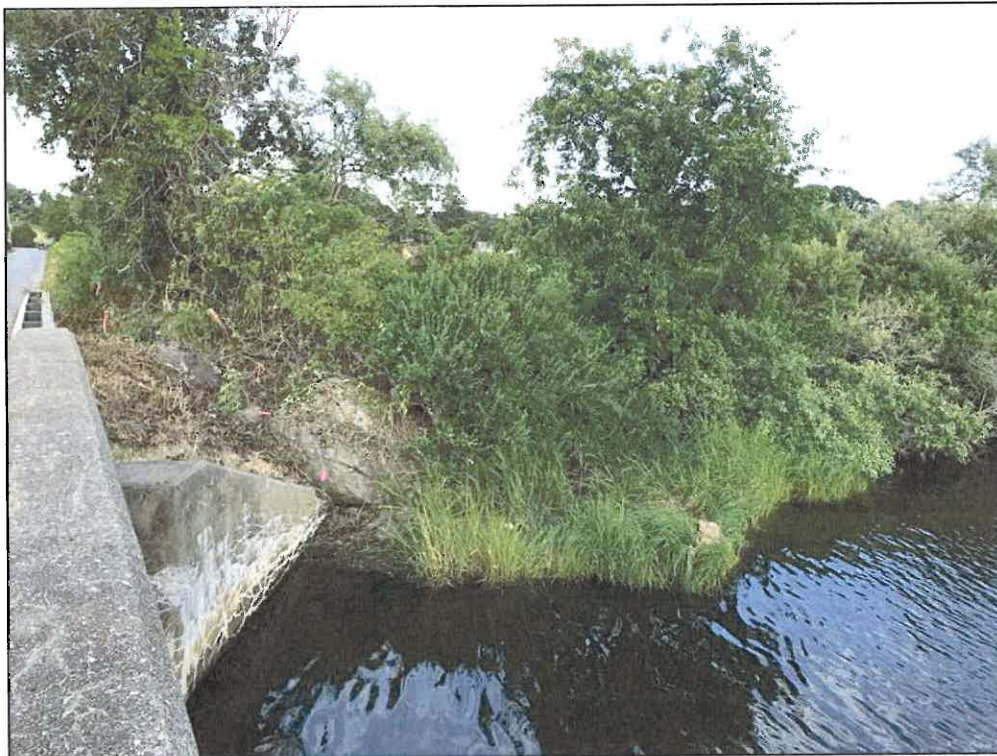
Photo No. 6: View of the eastern edge of Almy Creek. An ASSF (ASSF 200 series) extends from a roadside swale to the creek edge. A fringe of saltmarsh occupies the tidal shoreline.
