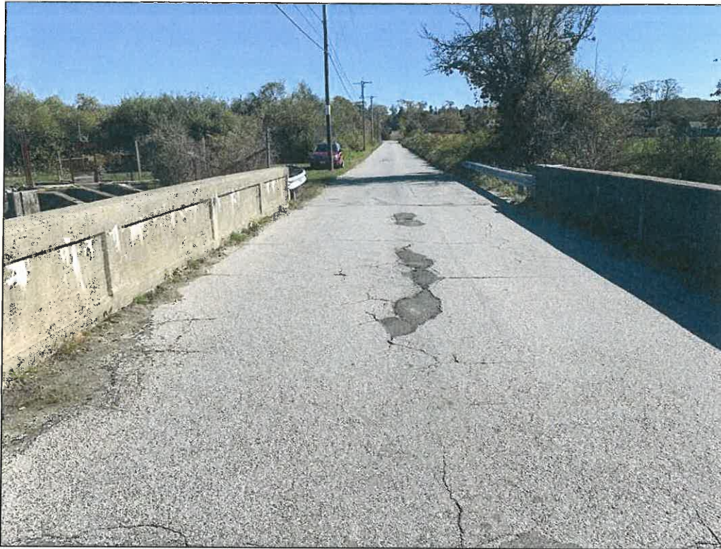
Photo No. 1: View of Pond Bridge Road and Nonquit Pond Bridge facing east.
