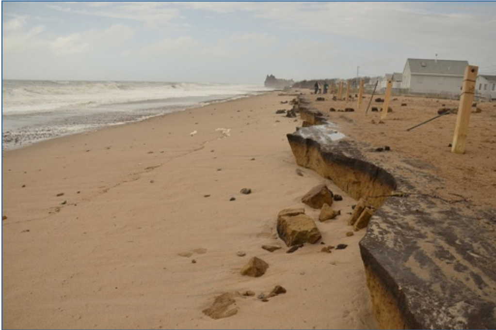
Extensive erosion in Matunuck, R.I. Tropical Storm Sandy caused severe erosion along the southern Rhode Island coast in 2012.
