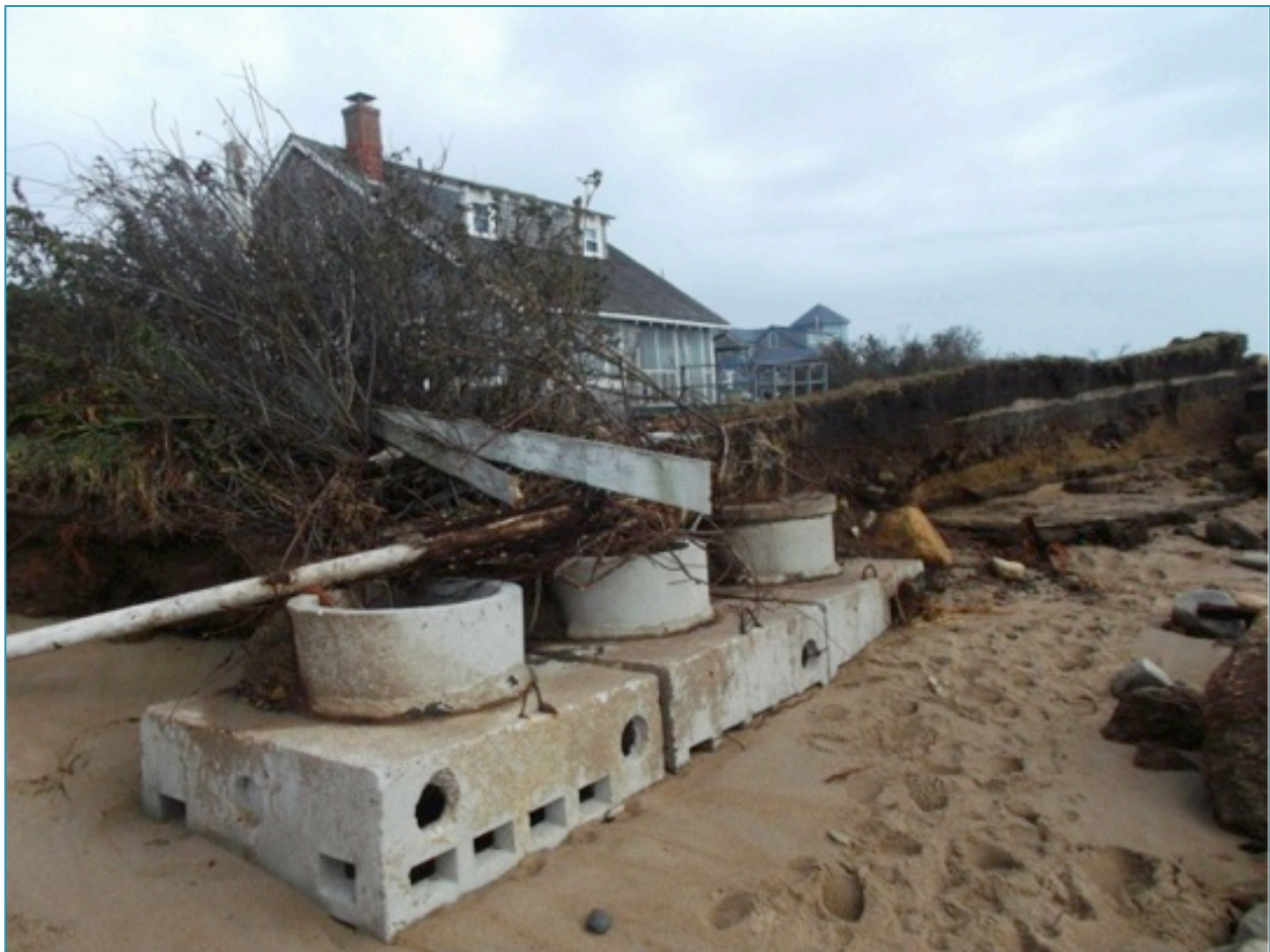
Exposed septic system: Erosion can uncover and damage septic systems during severe coastal storms.
