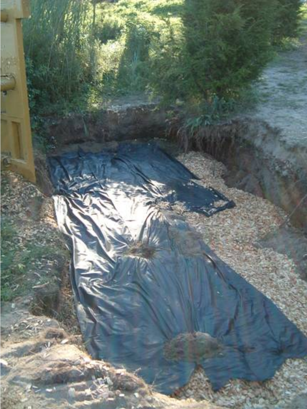
Fig. 5. A woodchip border during the backfill operation. The trench boxes have been removed, the trench pumped dry and backfilled with woodchips to about one foot above the water table. Landscaper cloth was used to prevent soil from penetrating into the woodchip media.
