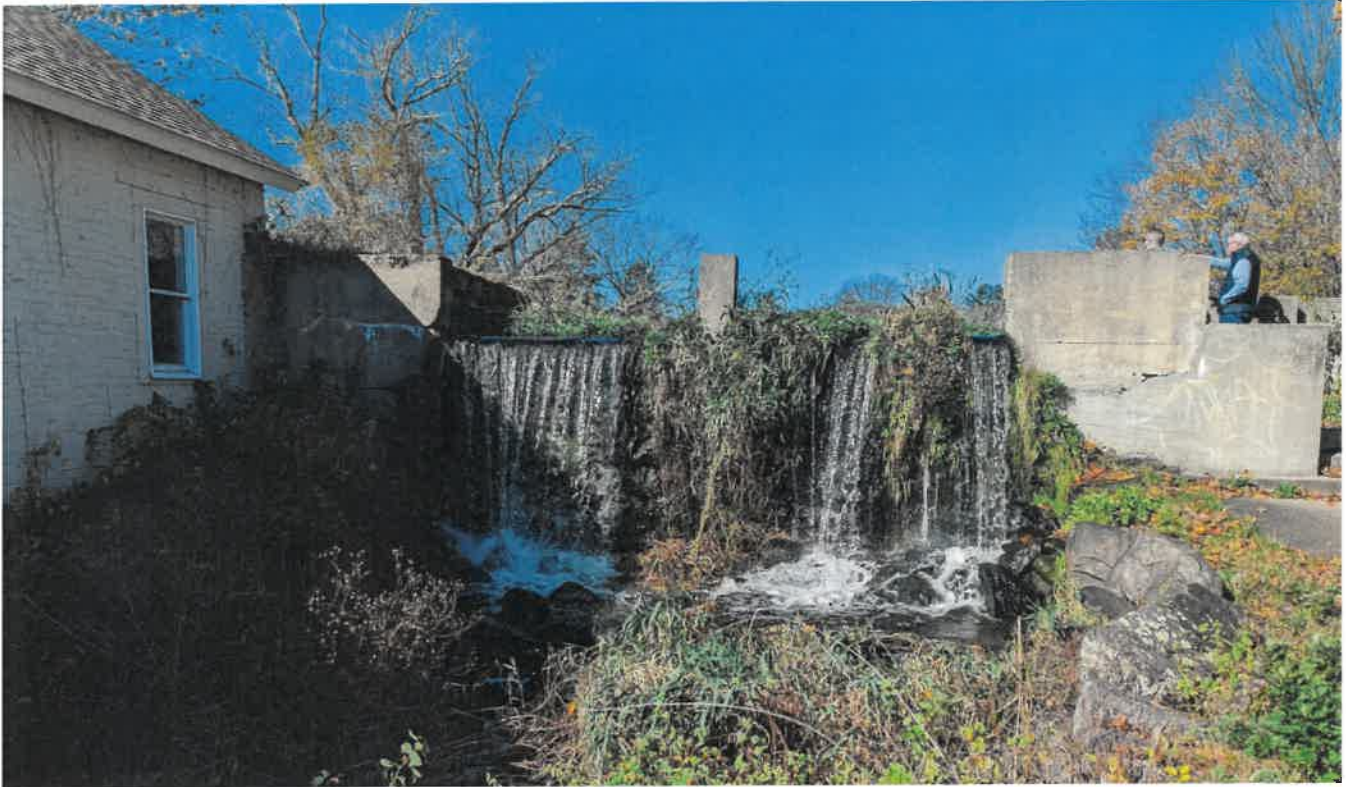
Figure 2: Photo taken during the November 8, 2022, site meeting of the Rodman Mill Dam spillway, within the Annaquatucket River in North Kingstown. Property owner Michael Baker is located in the top right corner of the photograph, describing site conditions.
