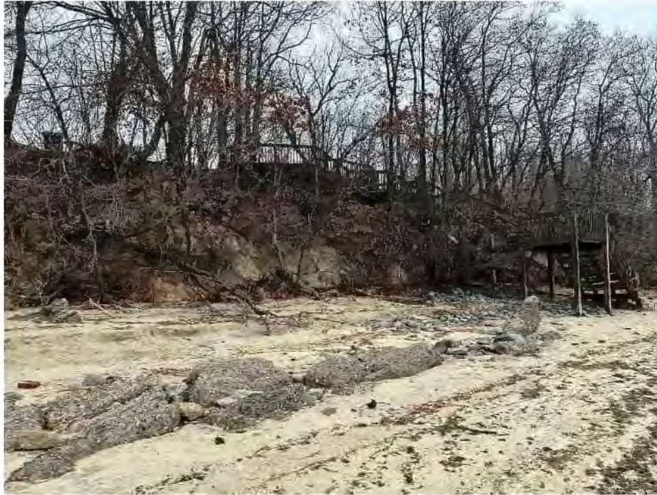
Photo 7: Significant erosion of slope, damaged stairs, downed trees on beach and unstable trees on slope from December 23, 2022 storm.
