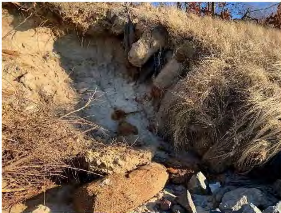
Photo 2: Damage/failed experimental coir log shoreline protection system.
