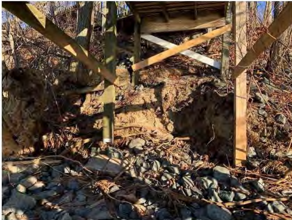
Photo 8: Damage to stairs from December 23, 2022 storm. Timber posts are no longer supported on any foundation system.
