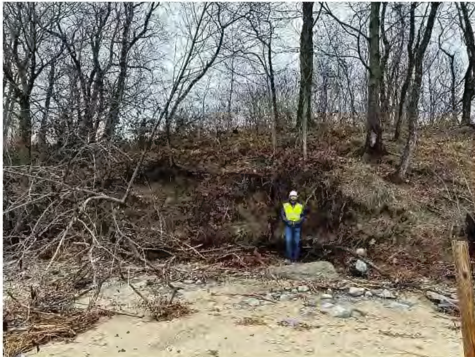
Photo 10: Significant erosion of slope, downed trees on beach and unstable trees on slope from December 23, 2022 storm. The individual in the photo is 6'-3" for reference.
