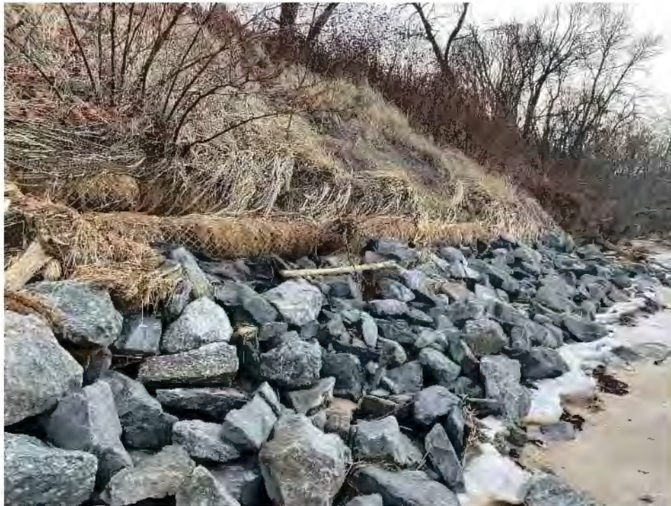
Photo 4: Damage to experimental coir log system. Note stones missing from below coir logs were deposited on the beach during the December 23, 2022 storm.
