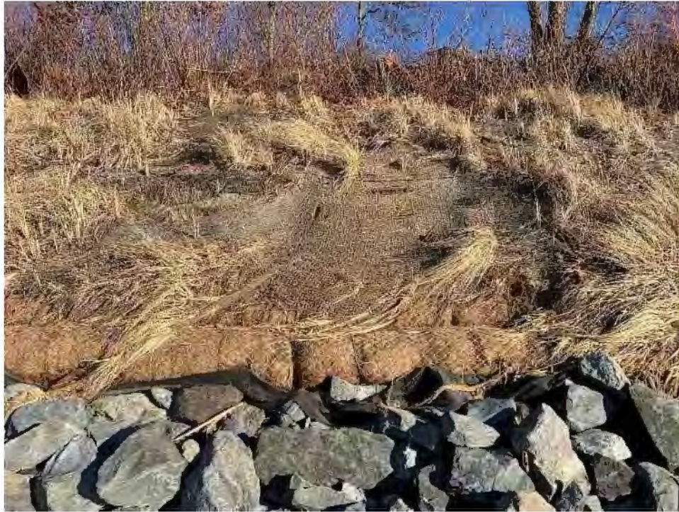
Photo 3: Damage to experimental coir log shoreline protection system.
