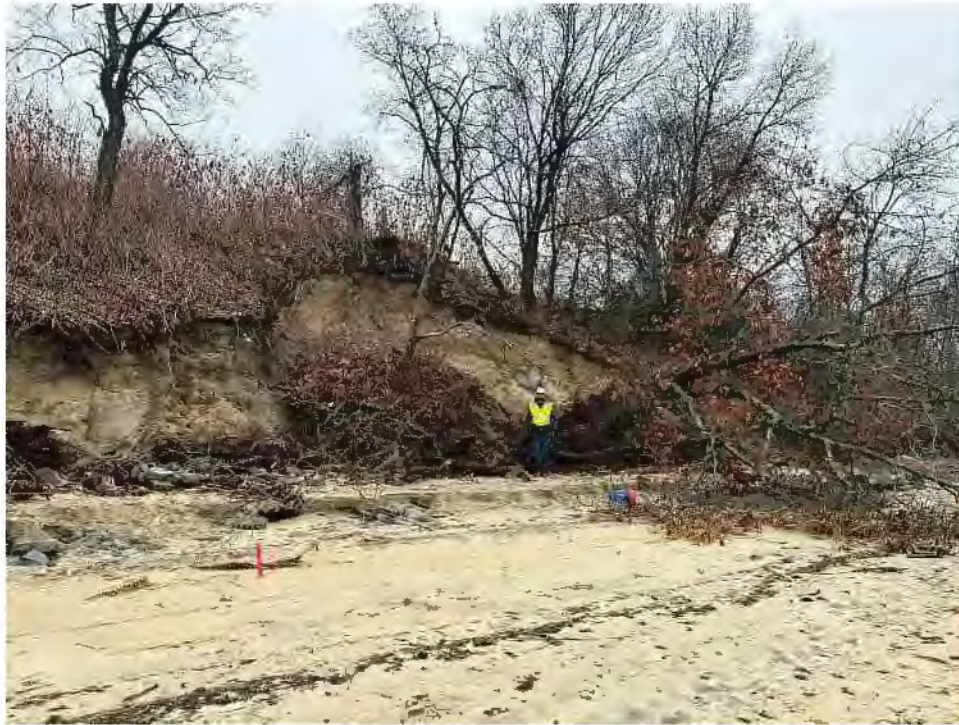
Photo 5: Significant erosion of slope, downed trees on beach and unstable trees on slope from December 23, 2022 storm. The individual in the photo is 6'-3" for reference.
