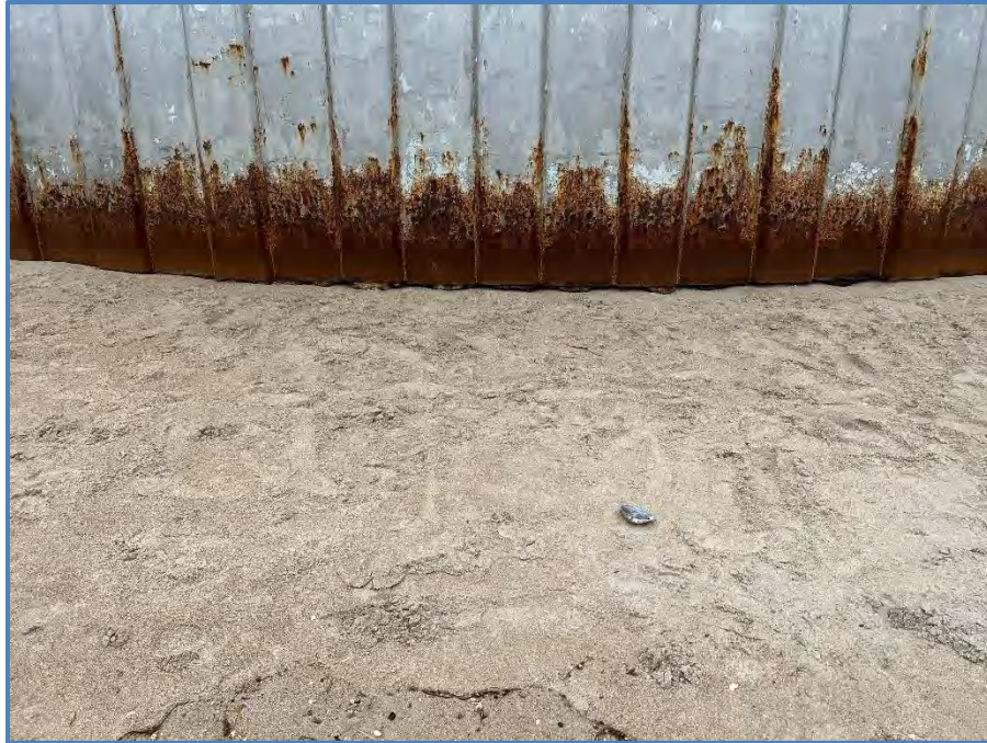
Figure 15: Exposed Toe of Pan Over sheeting at Time of Site Visit
