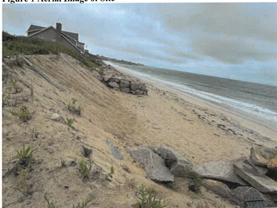
Figure 2 Image of existing gap in revetment
