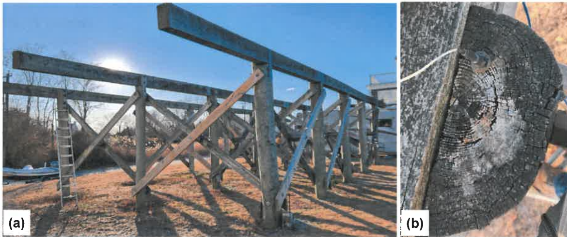
Figure 1. (a) Image of the Existing 256 Shawomet Ave Property. (b) Example Imagery of the Pile Head and Instrumented Accelerometer.
