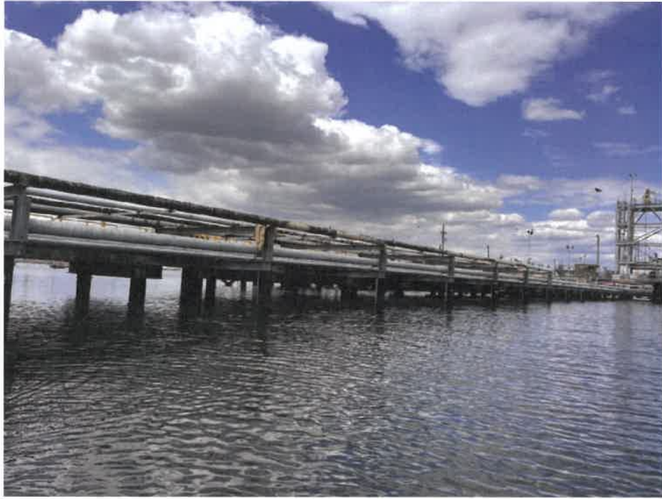
Photo 15: Southern steel pipe rack.
