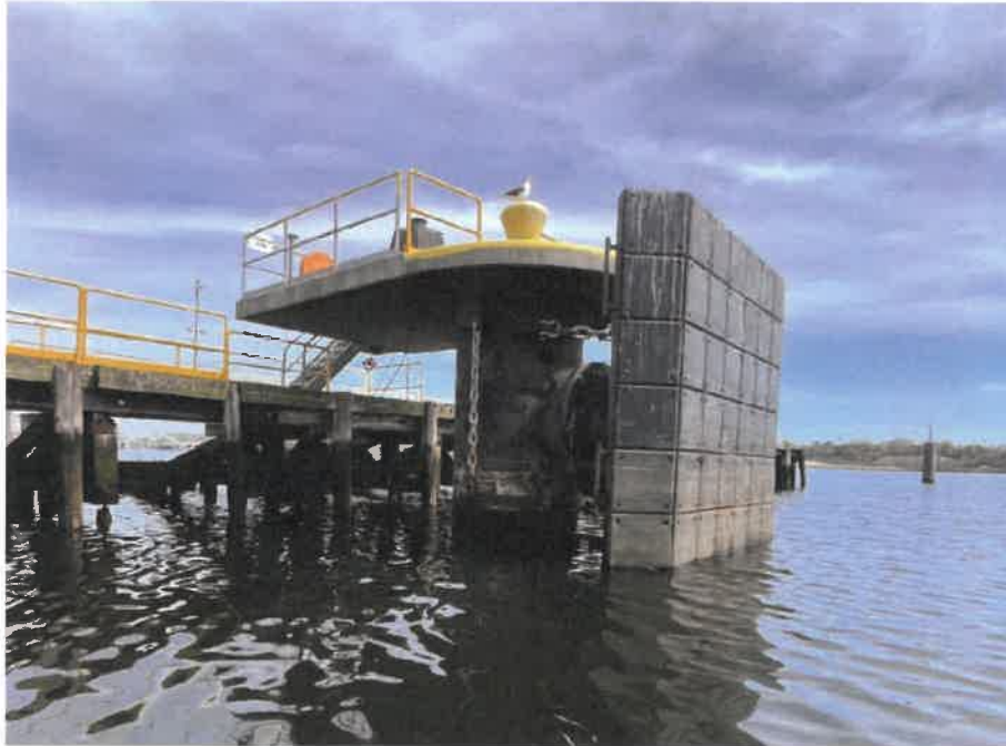
Photo 7: Steel monopile supported concrete mooring dolphin MD5. (Typical configuration for MD5 & MD6)
