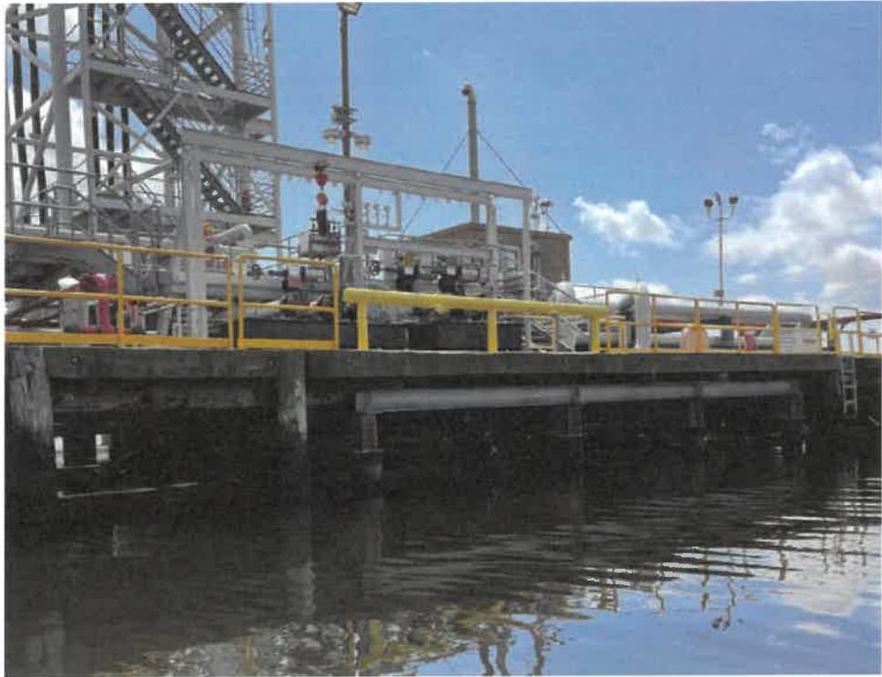
Photo 13: Barge hose platform.
