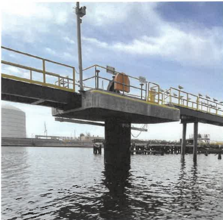
Photo 2: Steel monopile supported concrete mooring dolphin MD3. (Typical configuration for MD1, MD2, MD3 & MD4)
