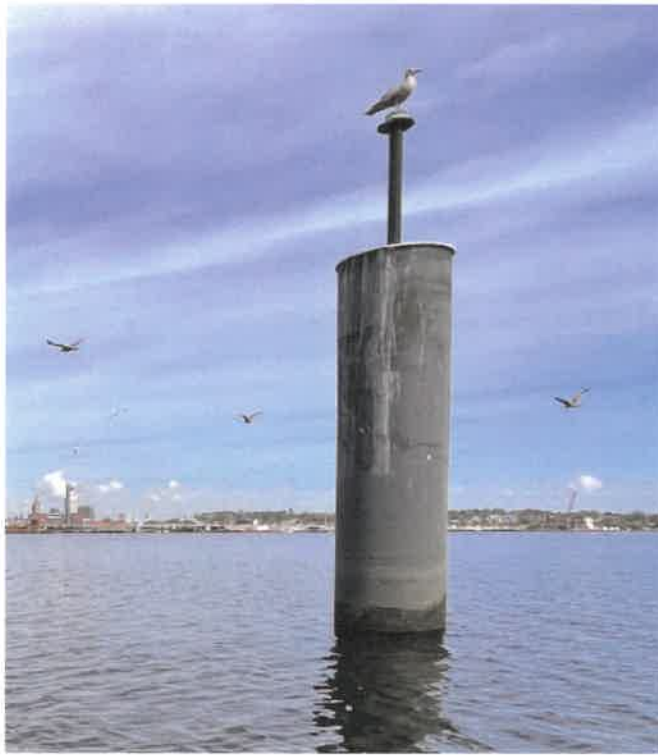
Photo 11: Property marker pile. (Typical configuration)
