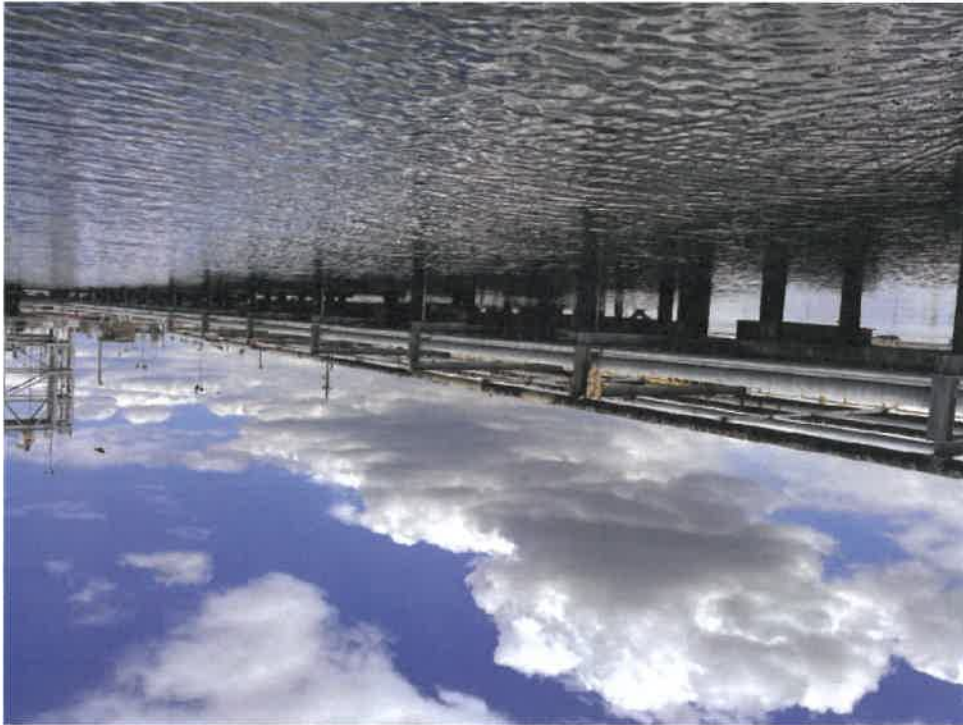
Photo 15: Southern steel pipe rack.
