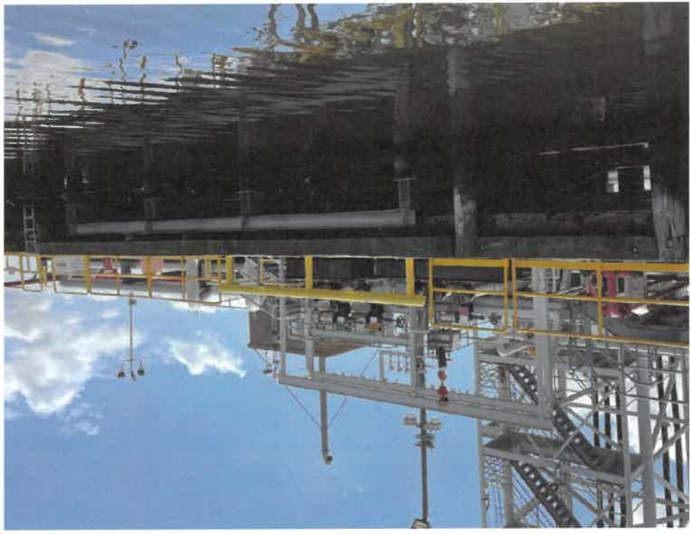
Photo 13: Barge hose platform.
