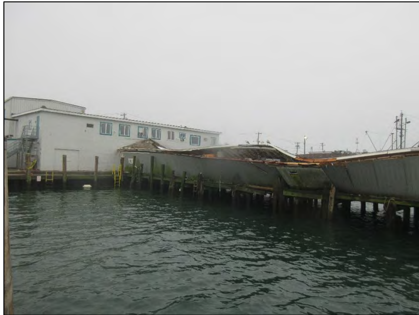
Photo 3: Prior to construction the building collapsed due to a snowstorm in March of 2023. The pier at this time is not in operation.
