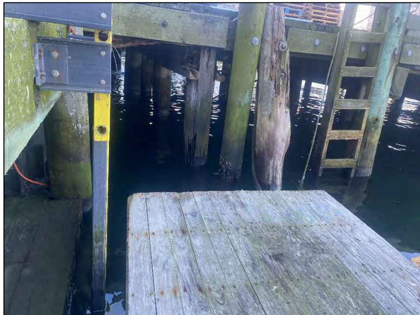
Photo 2: Support piles splintering and/or necking exhibiting signs that the piles are beyond the serviceable life in the current condition
