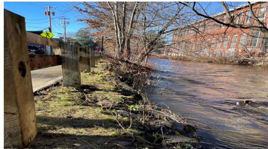
FIGURE 1G – ERODED RIVERBANK ALONG BIKEPATH/SAN SOUCI DRIVE FACING UPSTREAM LOOKING WEST. PHOTO TAKEN AFTER DECEMBER 18, 2023 RAINFALL EVENT.
