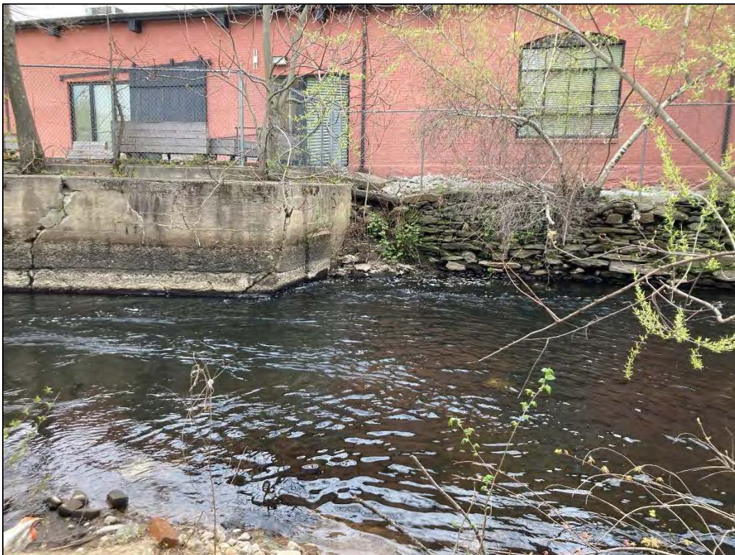
Photo 8: Face of cracked retaining wall perpendicular to flow, looking east (19 April 2023)
