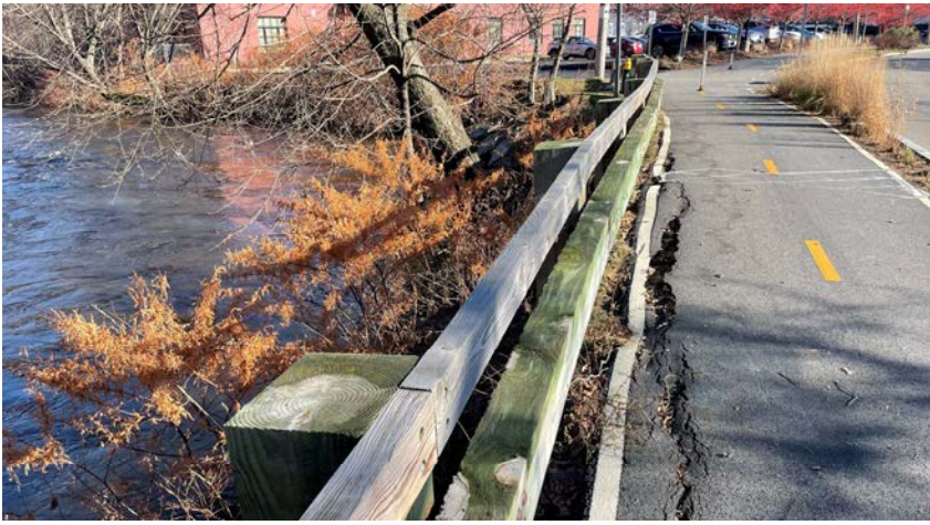
FIGURE 1A – SEPARATED BIKE PATH (WOONASQUATUCKET RIVER GRENWAY SPUR) ALONG SAN SOUCI DRIVE. SINKING AND CRACKING OF PAVEMENT AS A RESULT OF BANK EROSION VISIBLE. PHOTO TAKEN AFTER DECEMBER 18, 2023 RAINFALL EVENT.
