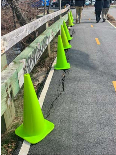
FIGURE 1A – BIKE PATH ALONG SAN SOUCI DRIVE SHOWING EXTENT OF PAVEMENT CRACKING. PEMA PLACED CONES ON PATH FOR SAFETY MEASURE. FACING EAST.
