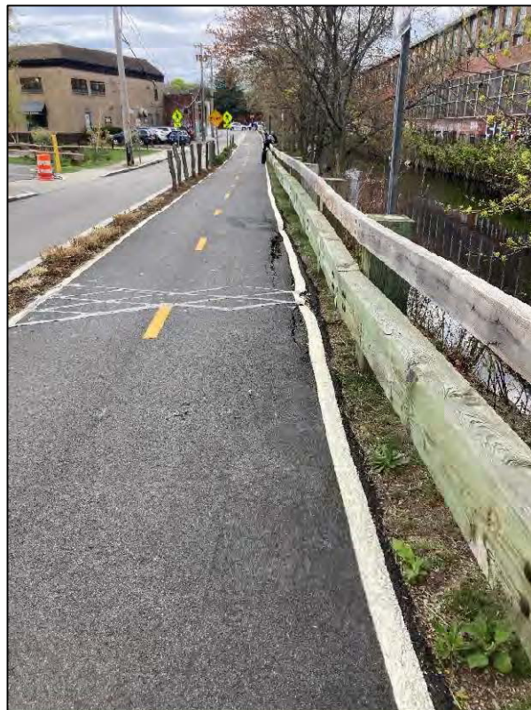
Photo 4: San Souci Drive and cracked asphalt on bike path, looking west (19 April 2023)
