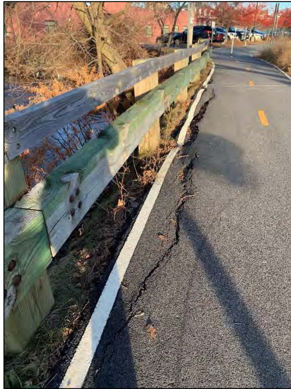
Photo 5: Cracked asphalt on bike path, looking east (11 November 2023)
