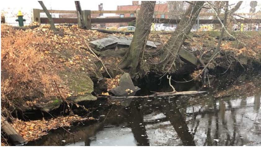
FIGURE 1B – VIEW FROM RIVER OF AN ADJACENT AREA. TREE ROOTS ARE EXPOSED/UNDERCUT. THIS AREA IS ADJACENT TO BIKEPATH AND SAN SOUCI DRIVE.
