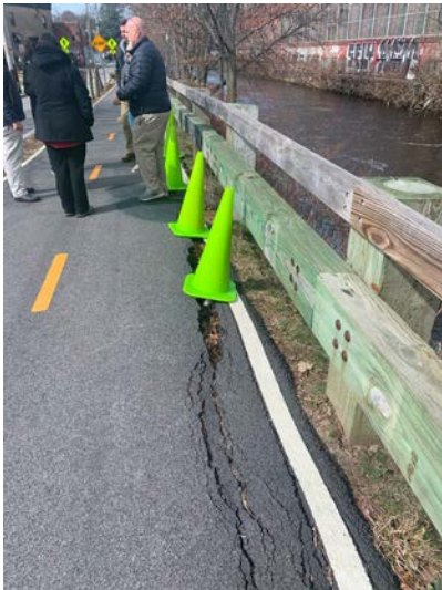
FIGURE 1B – BIKE PATH ALONG SAN SOUCI DRIVE SHOWING EXTENT OF PAVEMENT CRACKING. PEMA PLACED CONES ON PATH FOR SAFETY MEASURE. FACING WEST.
