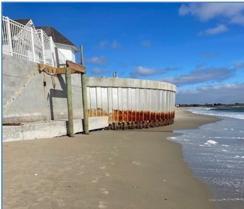
Figure 23: Scour along Seawall and Bulkhead after Storm
