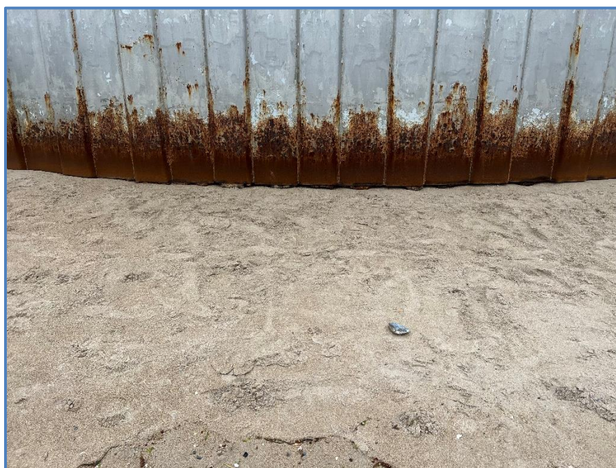
Figure 24: Exposed Toe of Pan Over sheeting at Time of Site Visit
