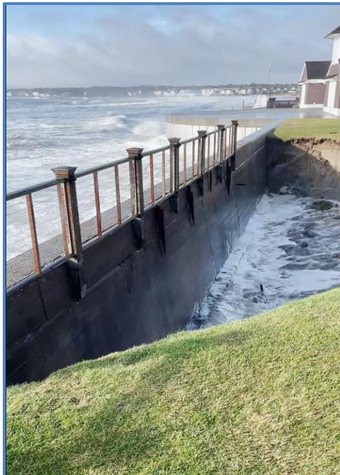
Figure 21: Area Undermined During Storm
