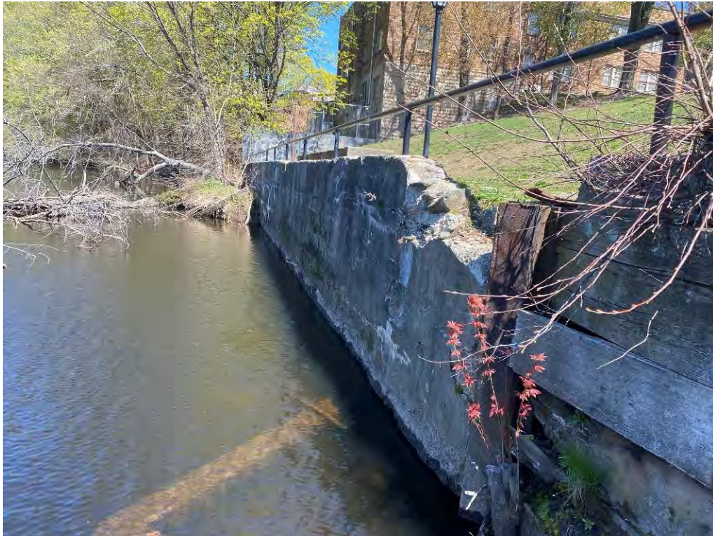
Photo 40: Concrete retaining wall north of former raceway channel Bay 4 intake, facing north (4/26/21)
