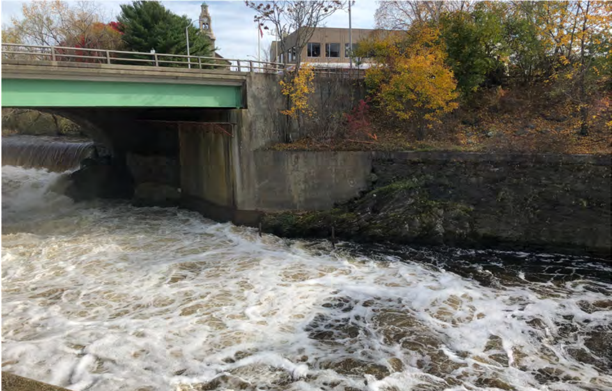
Former Apex parcel riverbank and Main Street bridge abutment, facing east (November 2018)
