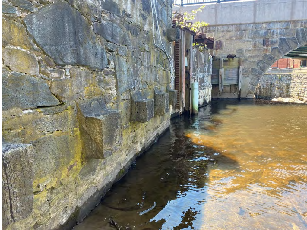
Downstream end of stone masonry retaining wall abutting Main Street Bridge, facing south (April 2021)
