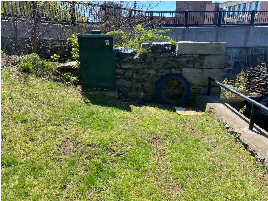
Electrical cabinet and vault adjacent to Main Street Bridge abutment (April 2021)
