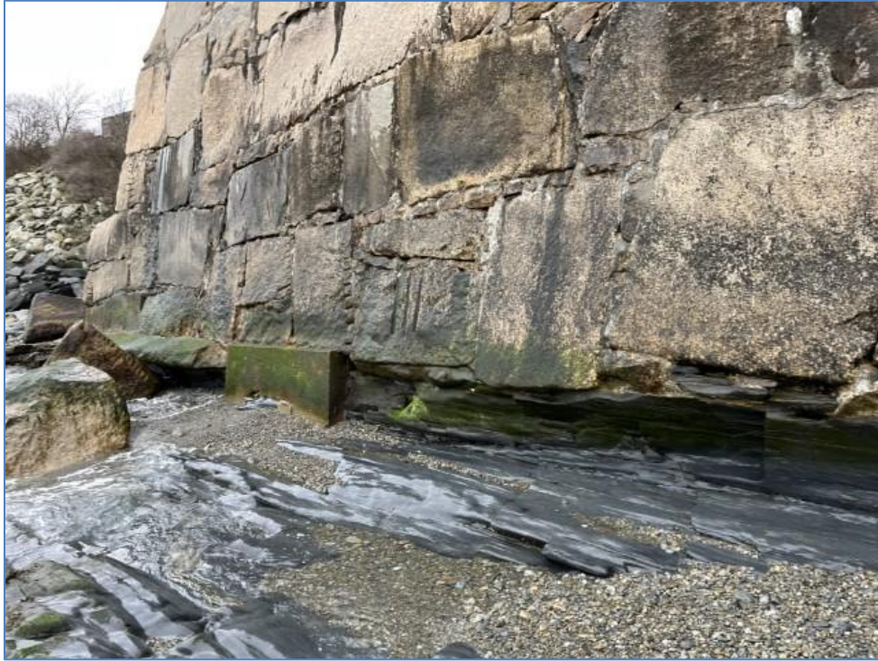
PHOTO 3: BEDROCK UNDERCUTTING AT THE TOE OF THE EXTANT GRANITE BLOCK WALL - LOOKING SOUTH
