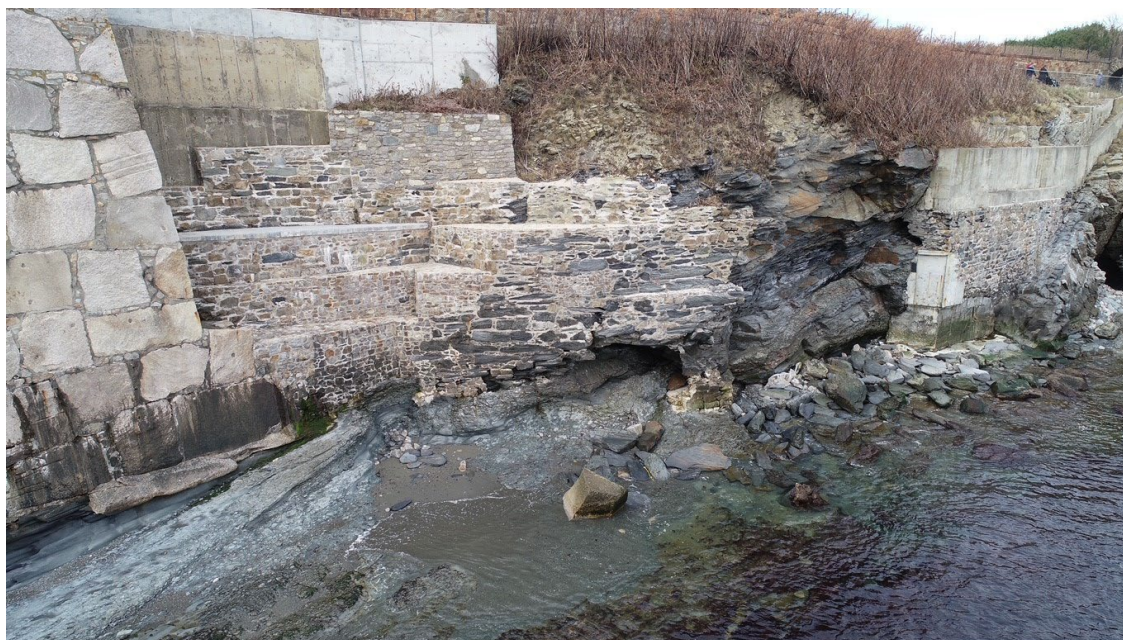
Photo 3: Slope along Cliff Walk in 1 st area that failed (prior to the failure) – note hole in masonry seawall along its base and also the bedding joints in the bedrock sloping toward the water
