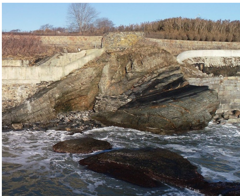
Photo 5: Overlook feature: note large eroded area between lower and middle bedrock section – given the sloping bedding plane the upper section will fail along this plane in the future which would cause failure of the bedrock, retaining wall and bridge supported above.
