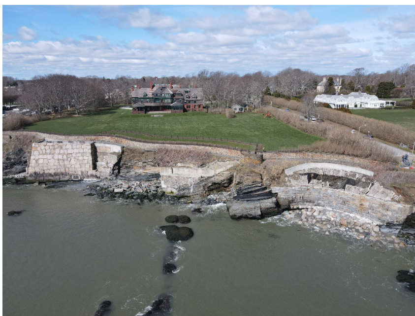
Photo 2: Slope along Cliff Walk proposed for repair – note failed areas & various wall generations
