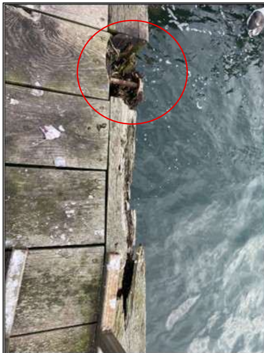
Photo No. 8.: Deterioration of timber chocks and observed damage to the timber support pile.
