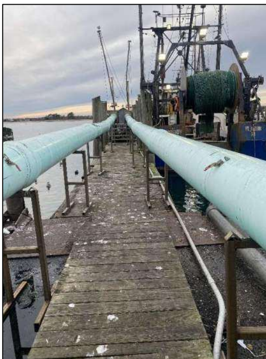
Photo No. 5.: View of the weathered decking of Pier 'JJ'.
