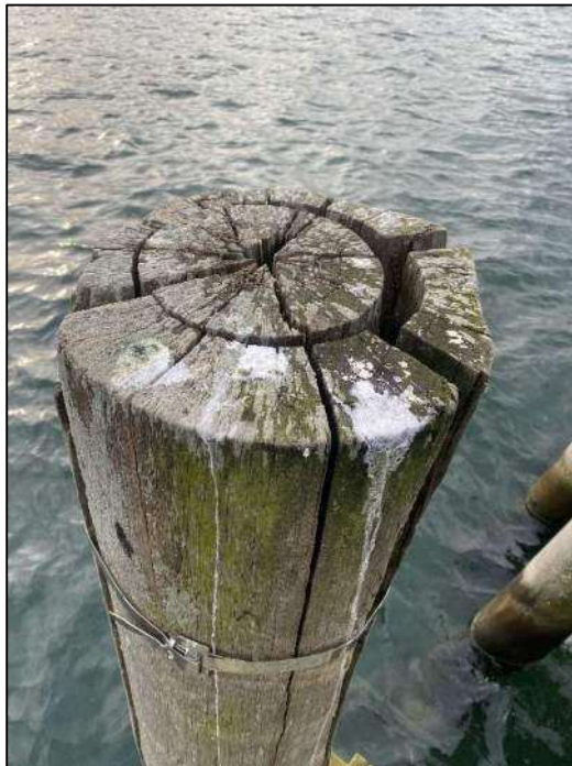
Photo No. 7.: Typical splitting of the fendering observed.
