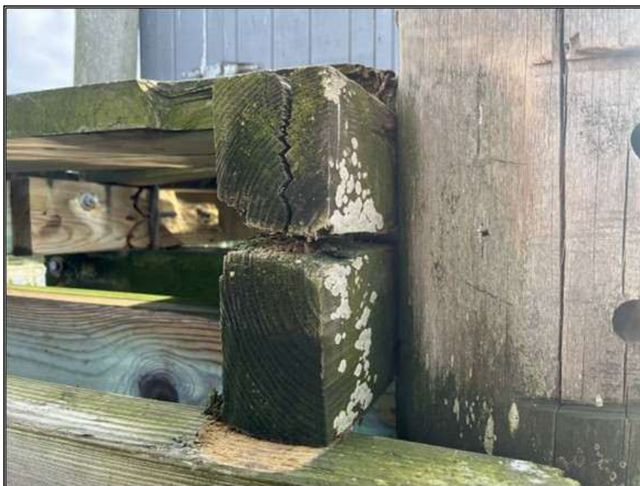
Photo No. 10.: Splitting of the end stringer of Pier 'JJ'.
