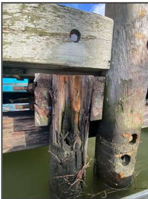
Photo No. 9.: Deterioration to the butt of the timber support piles, typical for 50% of observed support piles.
