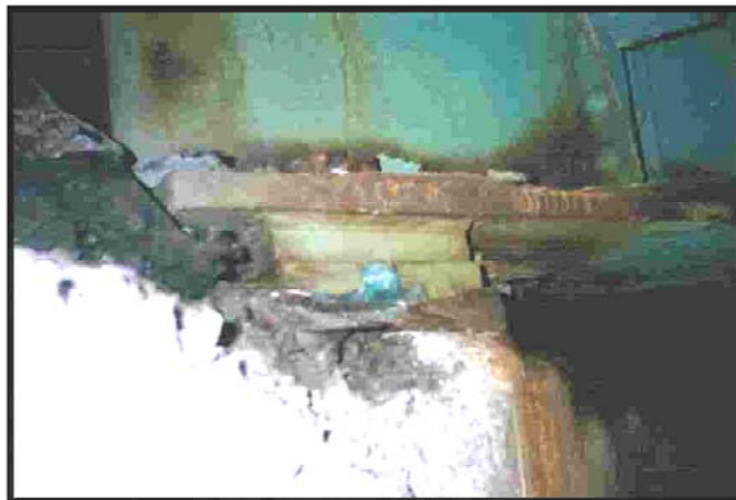
Beam seat deterioration
