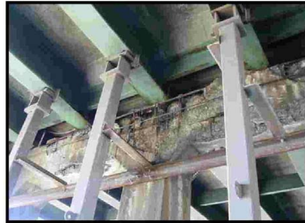
Exposed cap rebar
