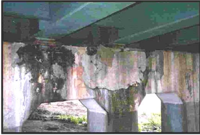
Typical pier deterioration
